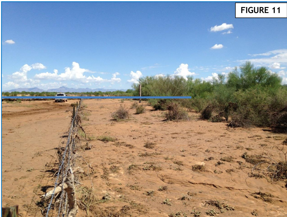
Rainbow Wash right overbank area (facing upstream), with approximate water level shown. Note debris line in fence which resulted from flow backing up at the highway culvert. (09/10/2014@13:22)
